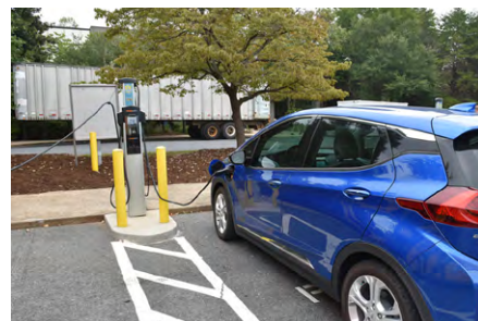
Electric Vehicle charging station. Source: National Rural Electric Coop.
